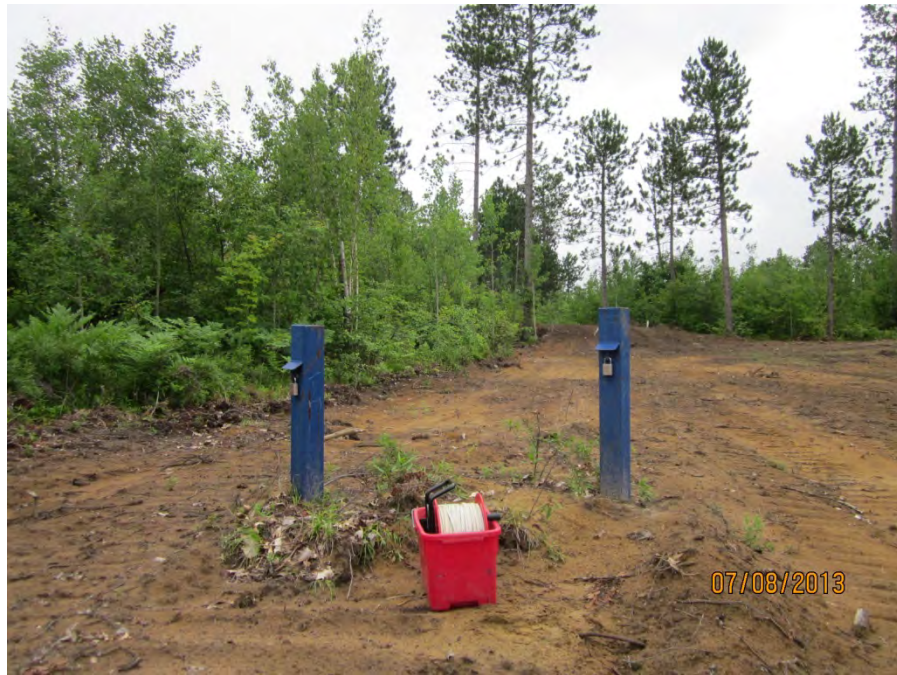
Photo 1 Groundwater monitoring wells BH1-I and BH1-II, July 2013
